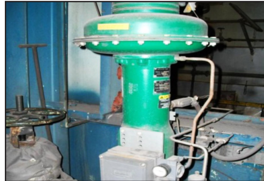
Valves, solenoids, and positioners require consistent air pressure to work efficiently.
